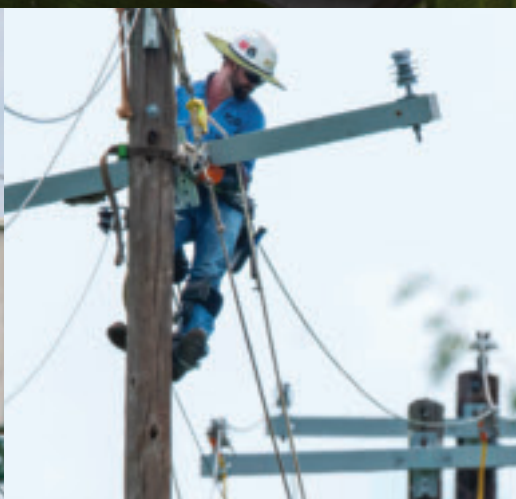
Our crews repaired lines in eastern Texas after powerful tornadoes and high-wind storms downed trees onto lines and caused widespread damage to the area.
