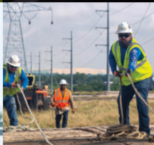
Our teams worked on new 125-foot transmission towers in Texas after devastating tornadoes. Dozens of towers spanning several miles of line needed to be replaced.
